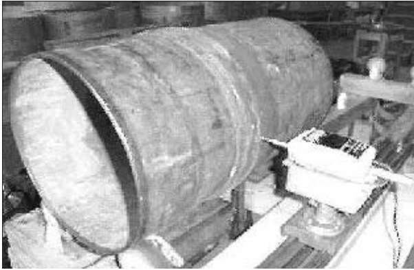
Fig. 13 Seismic strengthening of steel pipe joints using polymer composites. [Courtesy of Professor O'Rourke, Cornell University (Tutuncu, 2001)]
