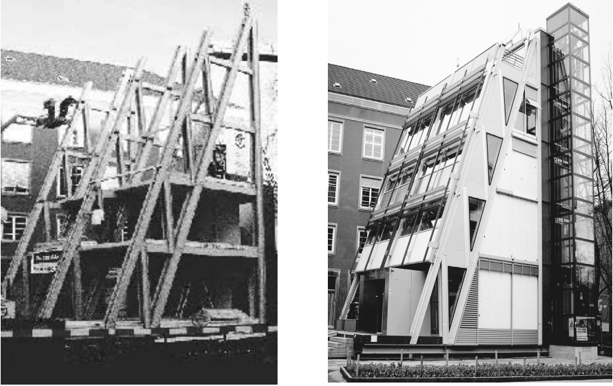
Fig. 46 All-composite "Eyecatcher" building in Switzerland: (a) pultruded frame skeletons and (b) the completed structure. (Courtesy of Fiberline Composites A/S)
