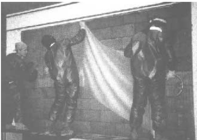
Fig. 16 Strengthening of unreinforced masonry walls using polymer composites. (Courtesy of Fyfe Co. LLC)
