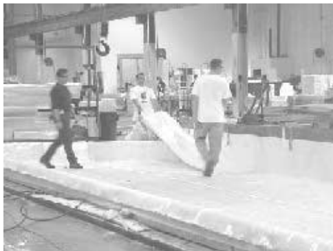
Fig. 50 Fabrication of the FRP composite bridge deck of NY 367 over Bentley Creek, Chemung County, New York. (Courtesy of New York DOT, Region 6, Hornell, NY)
