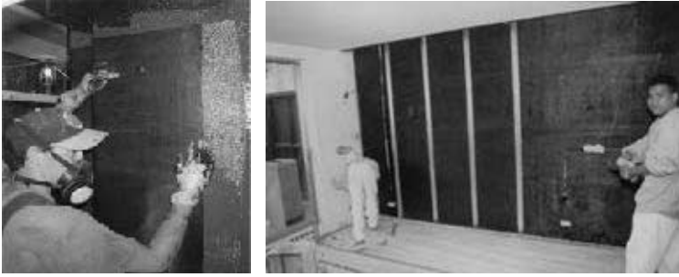
Fig. 10 Applications of composites for strengthening reinforced concrete shear walls. [Courtesy of Structural Composites Construction Inc. (SCCI)]
