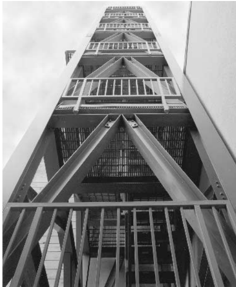
Fig. 47 Pultruded composites frame structure. (Courtesy of Strongwell Company)
